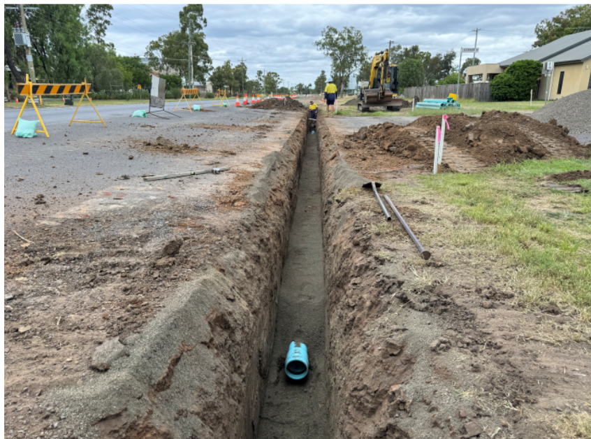
Open Cut 150mm PVC Water Main Replacement on Black Street & Leichhardt Ave Intersection Dalby
