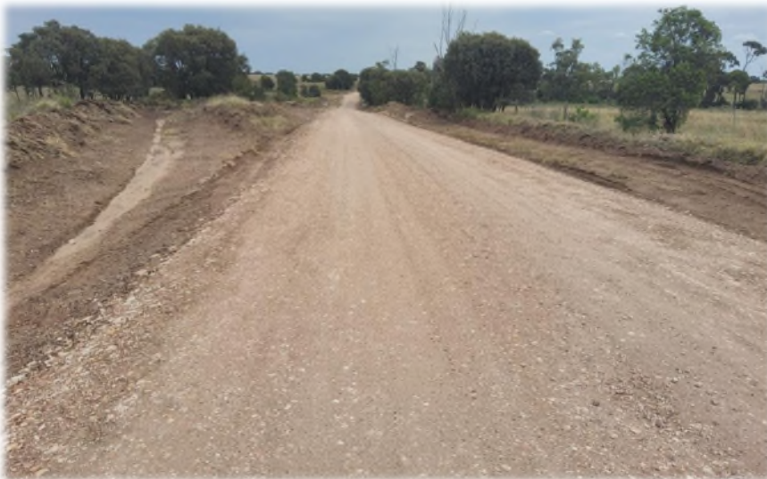
Completed Heavy Formation Grade with 50mm top-up on Burunga Lane from Flood Package 1
