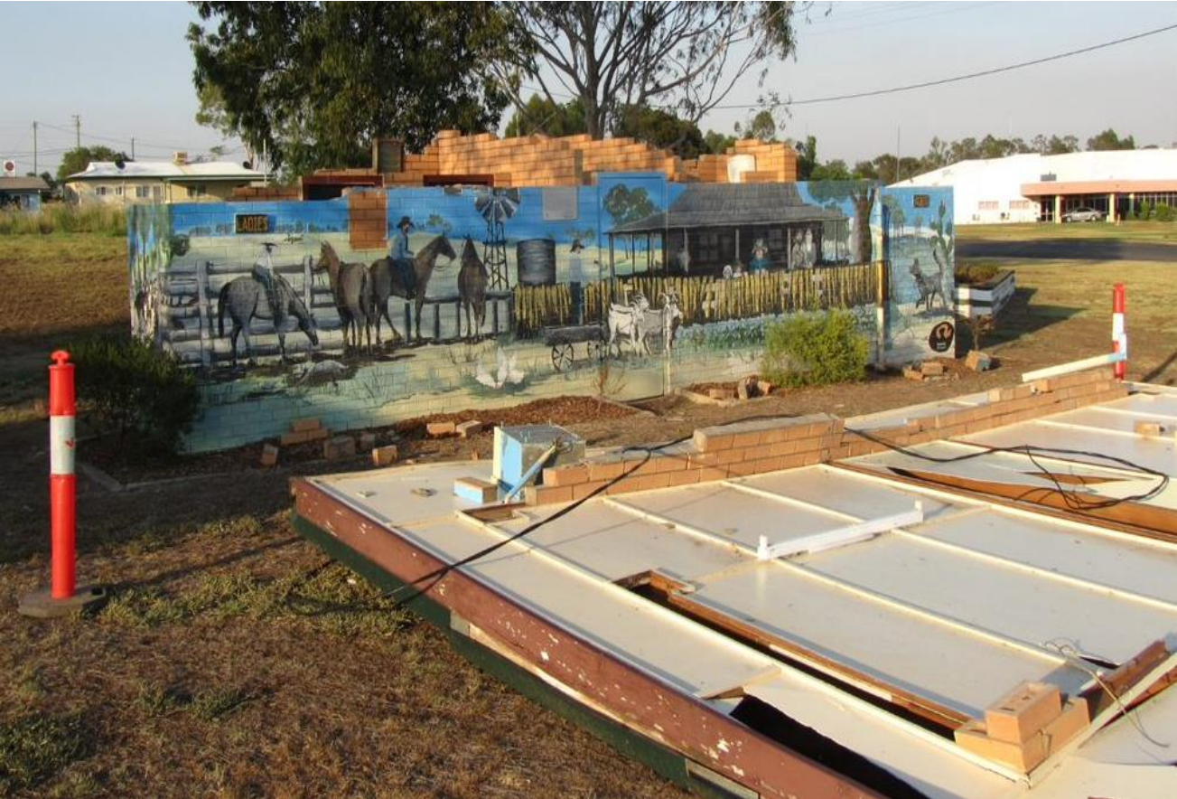
Attachment 2 - Damaged Amenity Block Corner Royds Street & Henderson Road Wandoan 2014
